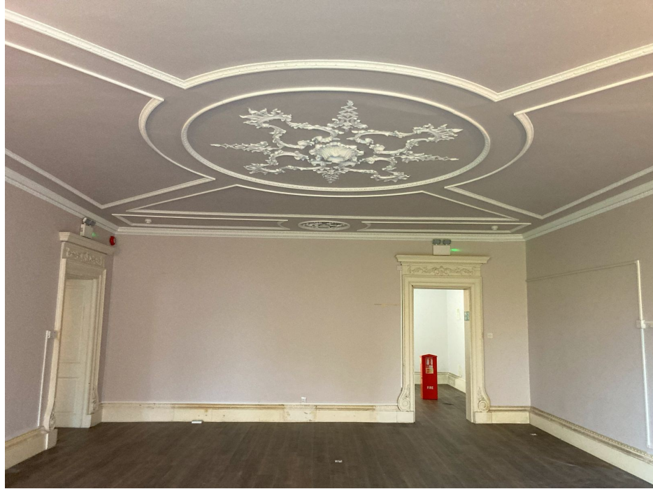
An empty Room 2 looking so much larger with the display cases having been temporarily removed and shows the ceiling plasterwork to maximum advantage.
